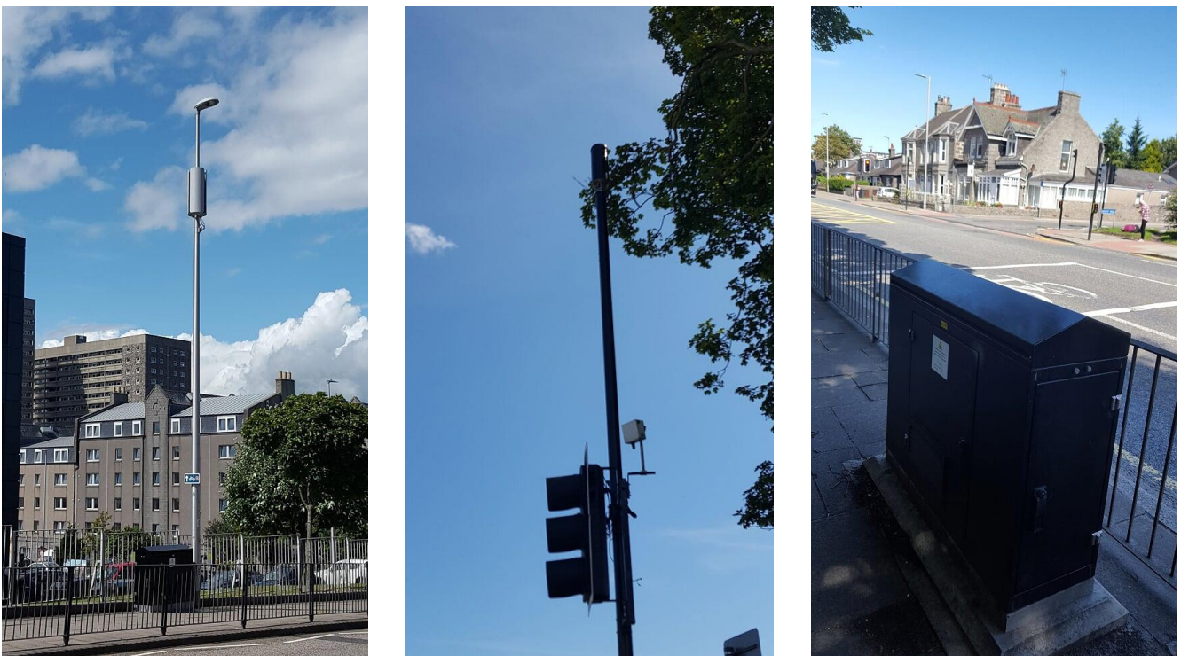
Figure 6 – Wireless Infrastructure Provider WIG have installed a neutral host network on a main road in Aberdeen. Mobile operator equipment is housed in standard green cabinets adjacent to street furniture
